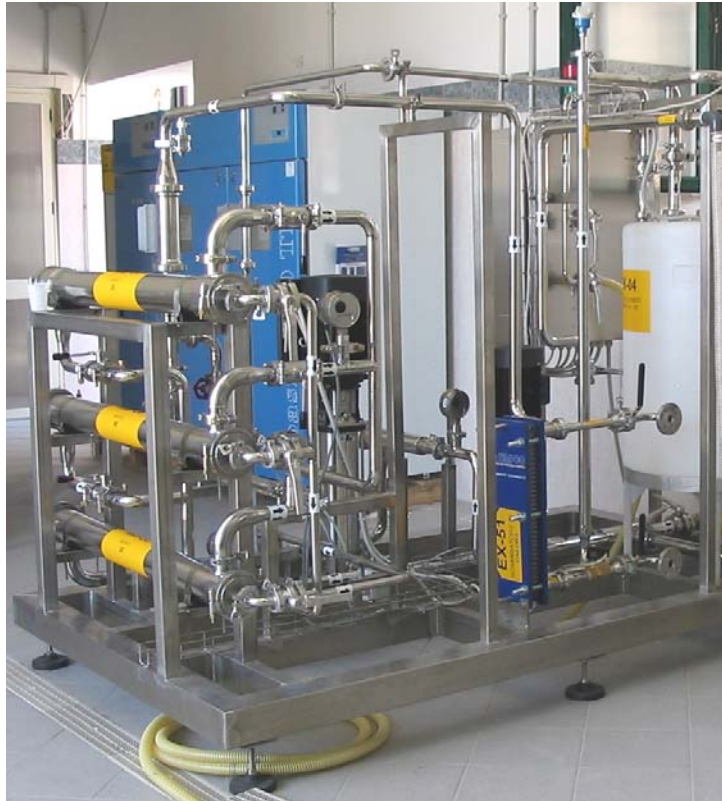
Figure 2. Pilot plant for OMWW treatment: polymeric ultrafiltration – nanofiltration – reverse osmosis section.
