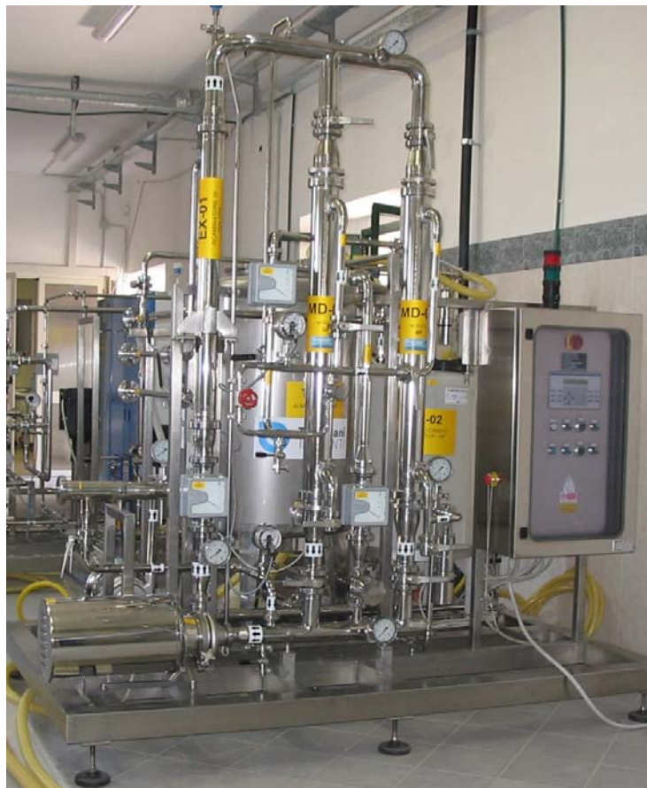
Figure 1. Pilot plant for OMWW treatment: ceramic microfiltration section.
